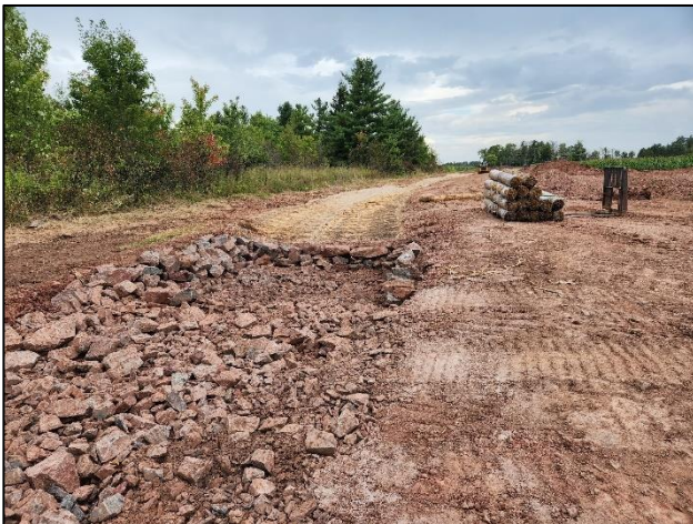
Construction of zuni bowl, which will allow water to ‘step down’ the newly stabilized ravine.
