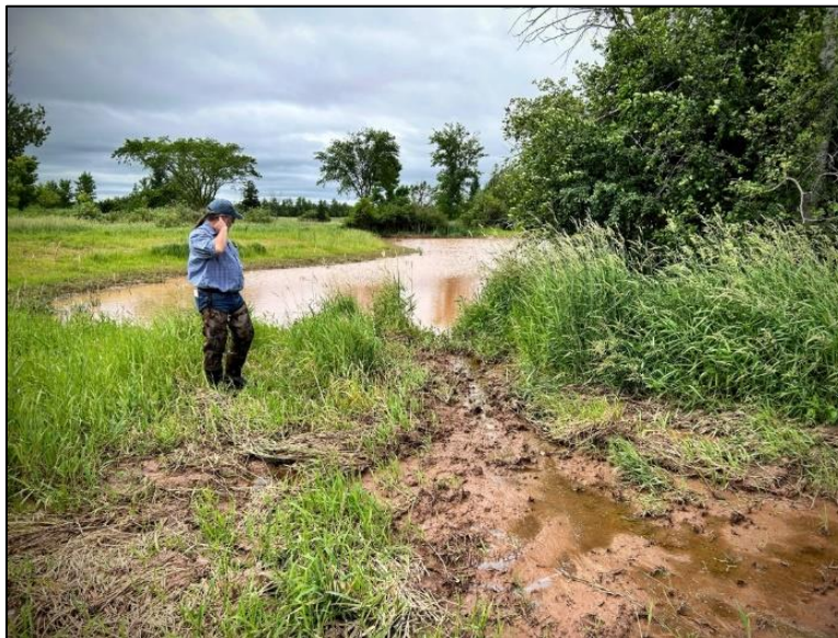
Headcuts are beginning to activate on main flow paths, near spillways that were installed at the Fischbach Wetland.
