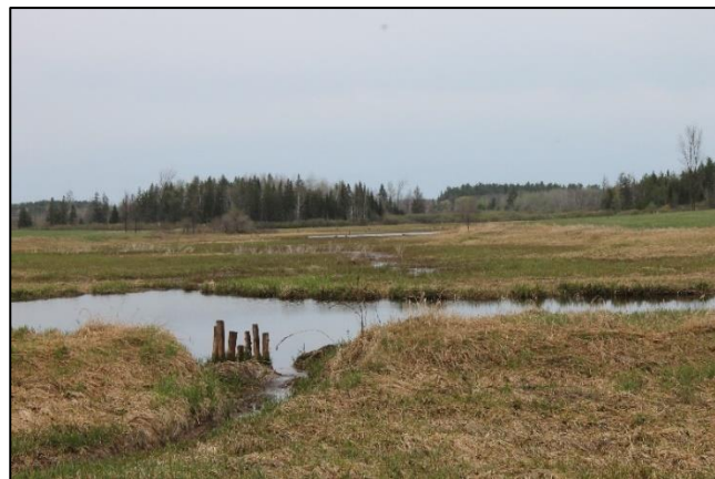
Aerial view of Mackey Wetlands (left) and close up view of the partially failed embankment (right).
