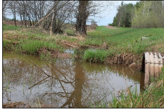
Sediment buildup before culvert, and water finding new paths.
