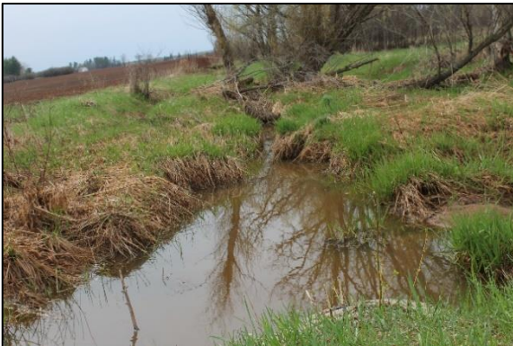
The channel leading to Berweger Culvert is overwhelmed with sediment, not allowing flow and debris passage.
