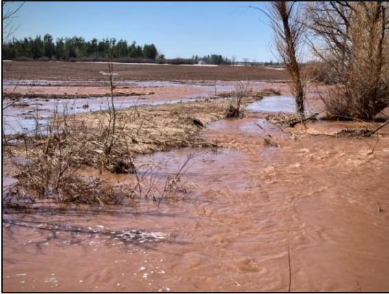
Backwatering before the Berweger Culvert after heavy rain. Water is finding new paths onto a farmed field and along road ditches.
