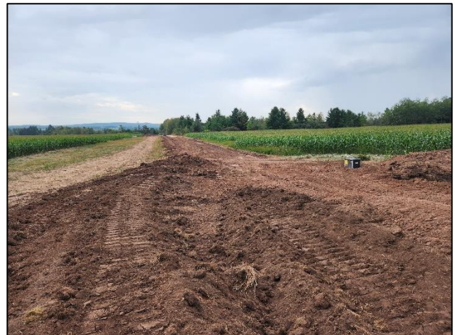
Water control structure visible at outlet of newly constructed scrape, and grassed waterway between cropped fields.
