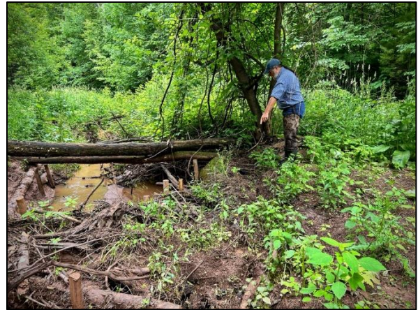
Flanking erosion around the sides of the PALs will require adjustments so flows do not bypass the structures.
